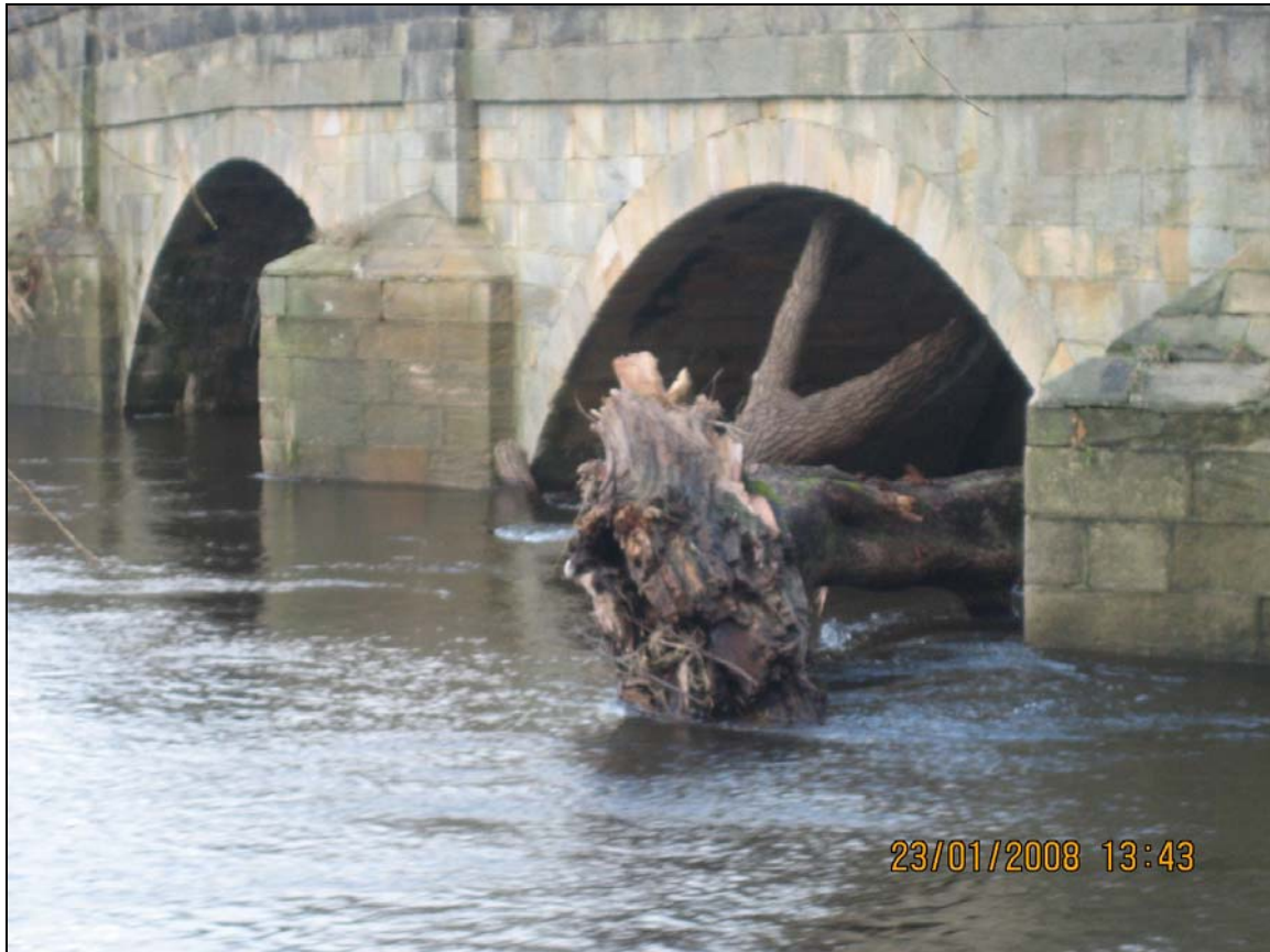
Tree trunk stuck under a Otley Bridge on the River Wharfe
