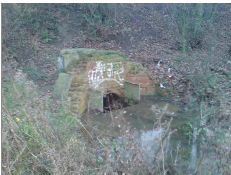
Difficult access to Stanhope Road culvert
