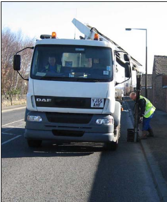
'Wet Spot' team at work with one of the new gully cleansing machines
